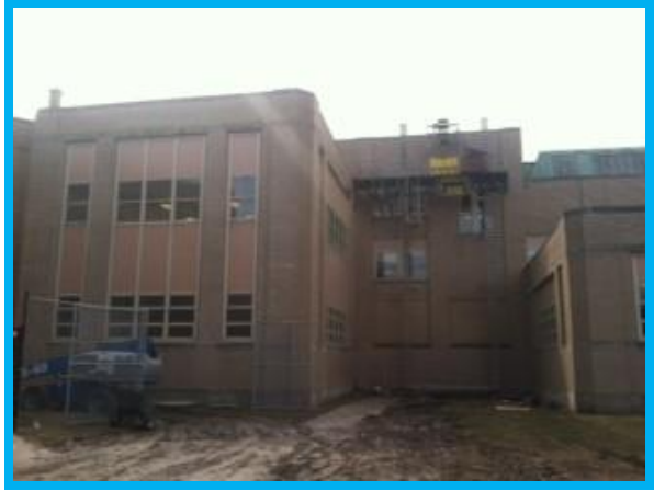
Architect of Record: DLR Group
